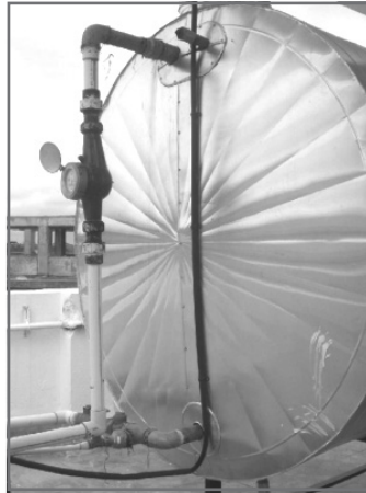
Water meter at hot water line
