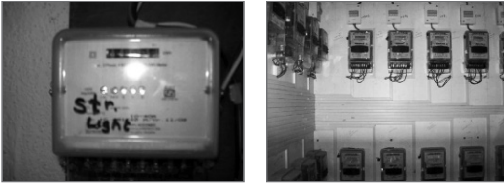
Picture 25: Photographs showing the energy meters installed
