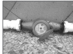
Water meter at swimming pool
