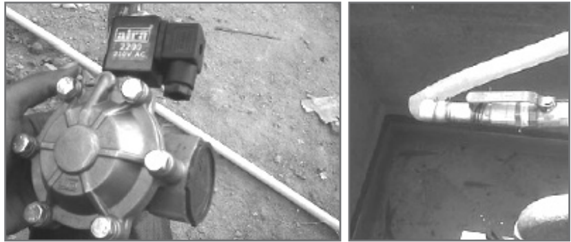
Picture 17: Photographs showing pressure regulating device & central shut off valve
